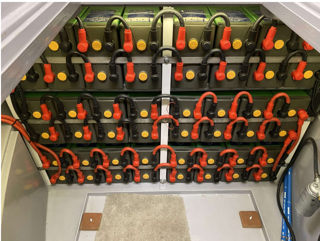
24 x 2V 800Ah Lead Carbon Batteries
